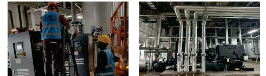
Compressor Heat Recovery System Retrofit
