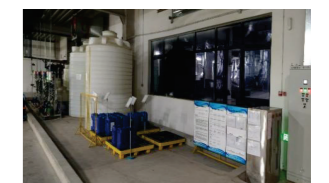
Field Equipment for Circulating Water Treatment
