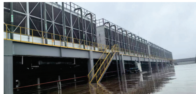
Condensate Reused in Cooling Towers
